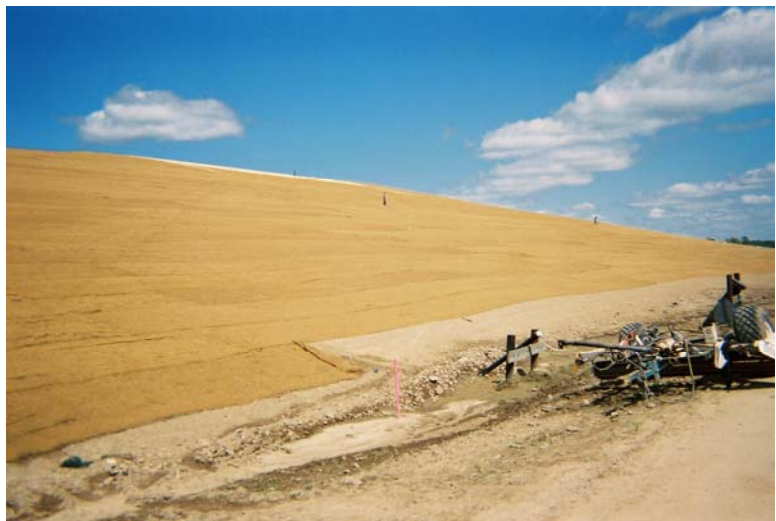
Landfill cap with erosion control blanket
