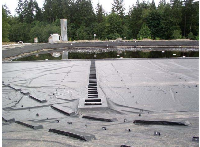
Olympic View Sanitary Landfill — Floating Leachate Cover, Port Orchard, WA USA
